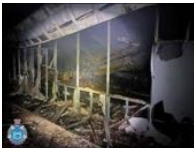
Yale Primary School was devastated by fire in March 2022.
